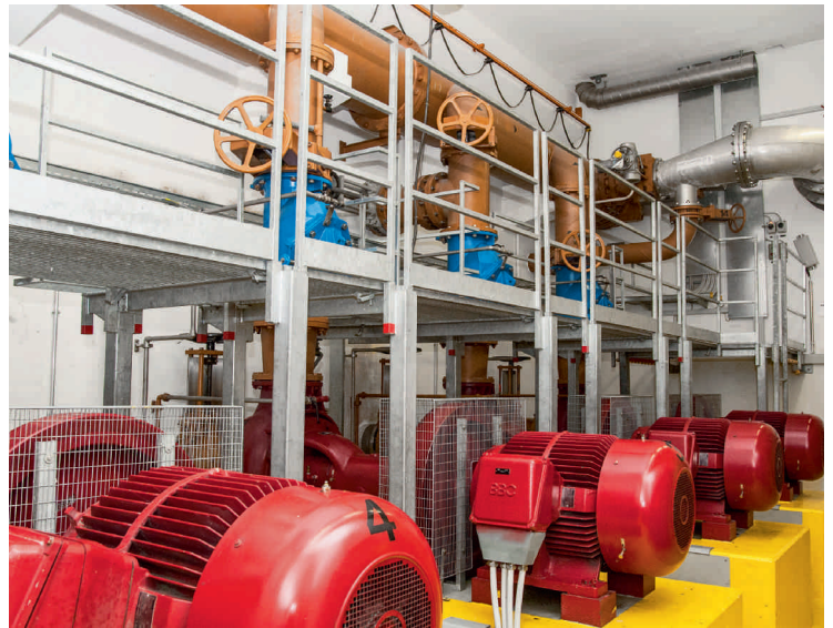
Fig. 1 Pumpstation Wollishofen / Station de pompage de Wollishofen
